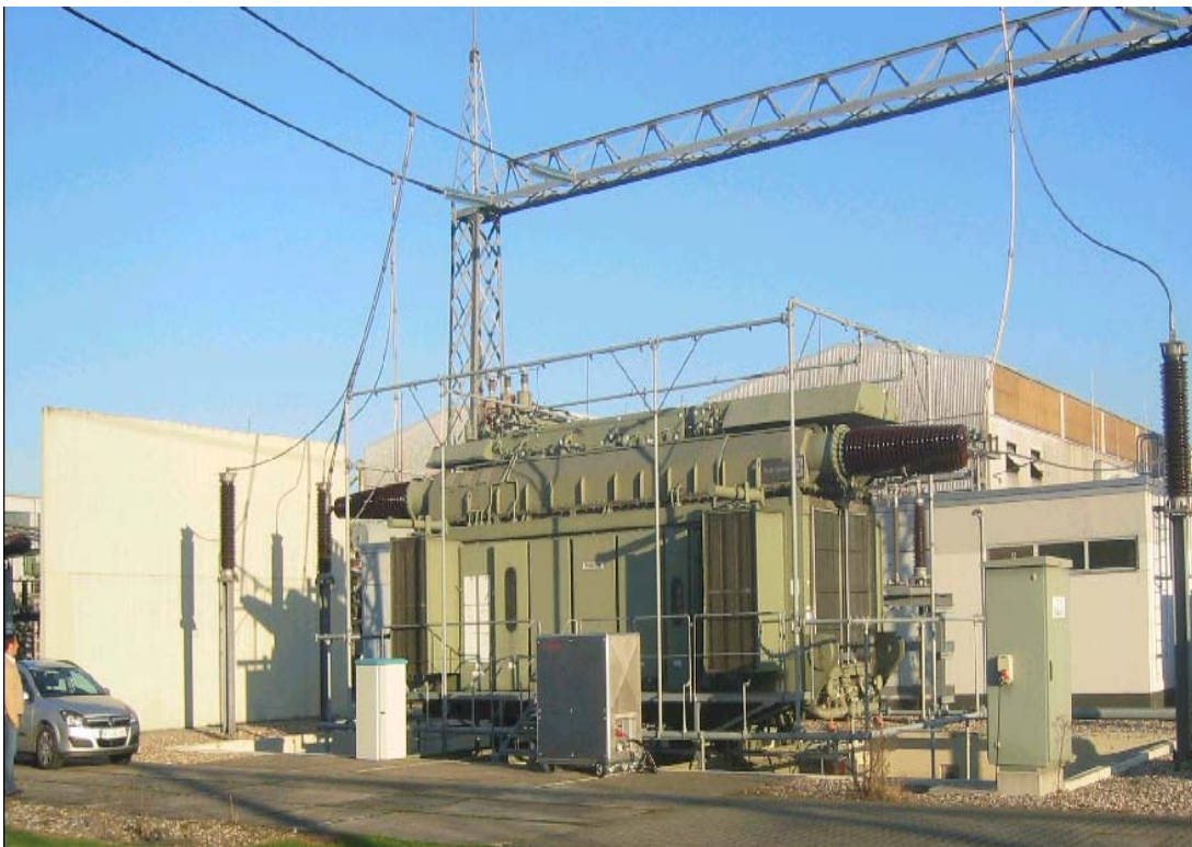
VS06 Climabox (and Online DGA)controlled life-extension of aged transformer
