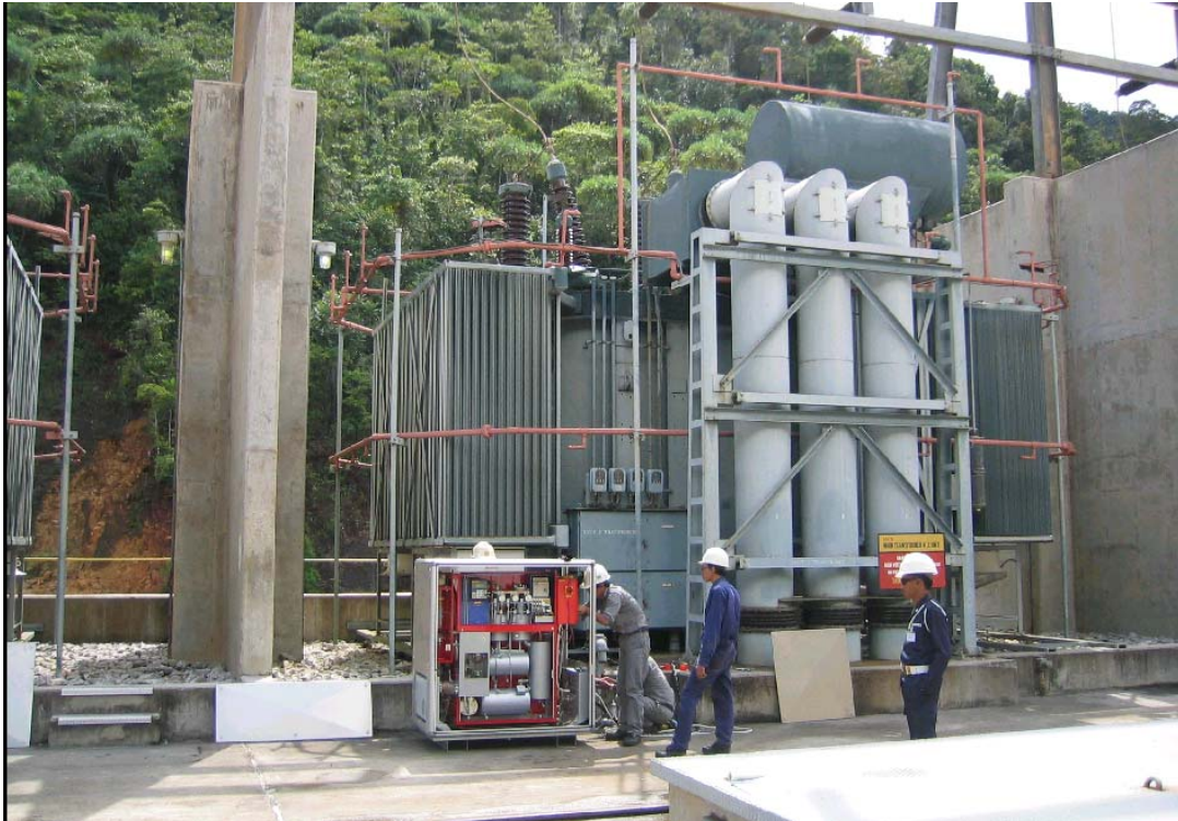
Germany: 250 MVA Transformer
