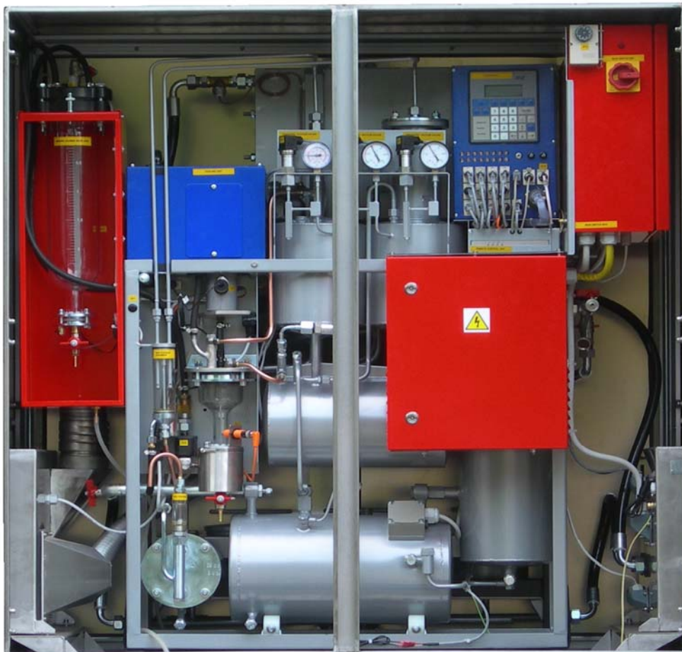
The internal layout of main components in separator VS-06 (front door open)
